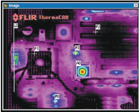
Figure 18.13 Heat analysis from thermal imaging camera.
