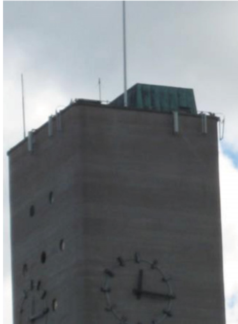
Figure 24.3 Installing antennas on the edge of a roof is a preferable way when looking the radiation safety, as we have here. Notice also the VHF-antenna on the short pole. Photo by Jouko Rautio.
