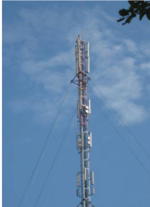
Figure 24.1 Antennas of mobile networks in a typical mast installation. Notice the tilting of the topmost antennas. Antenna height is enough to cause no RF radiation hazard to general public on the ground, but antenna fitters must take proper actions to avoid overexposure from neighboring antennas. Photo by Jouko Rautio.
