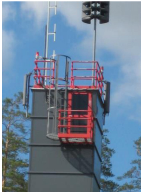
Figure 24.4 Not an ideal way for antenna installation. Part of the antenna is above the roof level and the radiation can penetrate people working on the roof. Fortunately in a sector antenna the back lobe is only about 1/100 of the main beam. Photo by Jouko Rautio.
