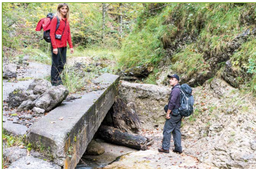
Fig. 44: Abandoned bridge on forest roads in wilderness zone.
