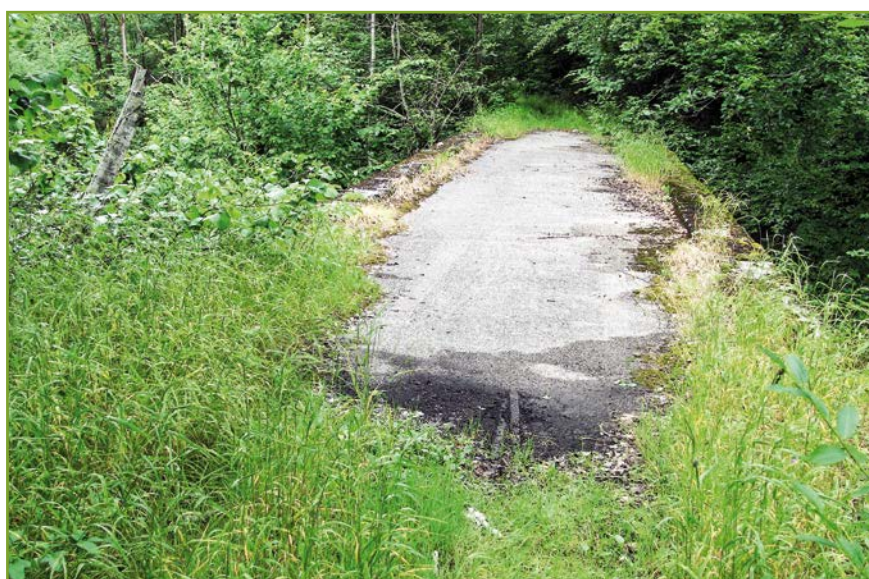
Fig. 50: The area also provides a unique example of long-term forest roads restoration.
