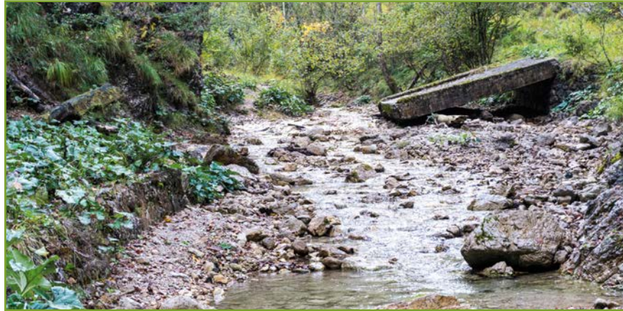
Fig. 84: Poor conditions of gravel roads limit motorized access to the wilderness zone.
