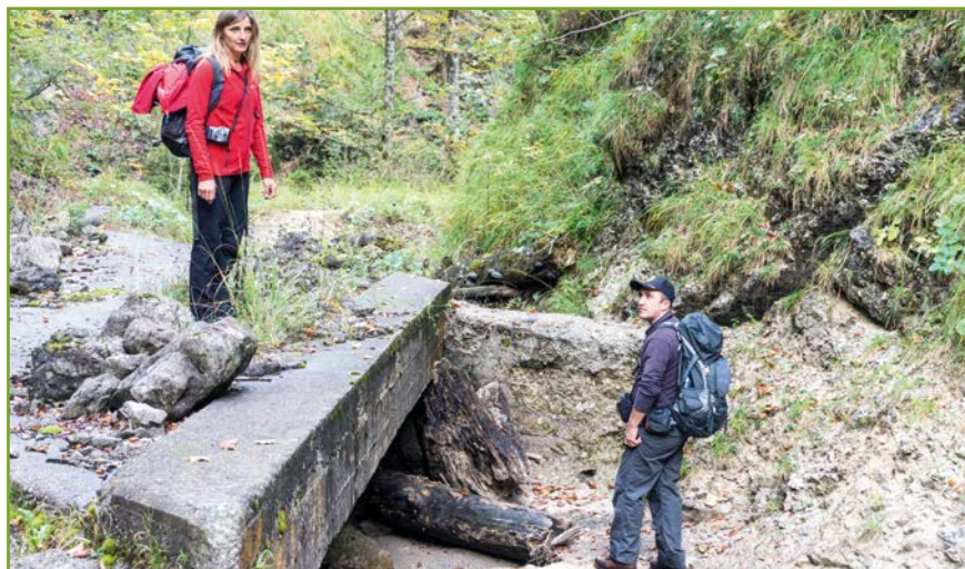
Fig. 82: Part of the restoration process is also abandoned and disused infrastructure that are located in the restoration zone.
